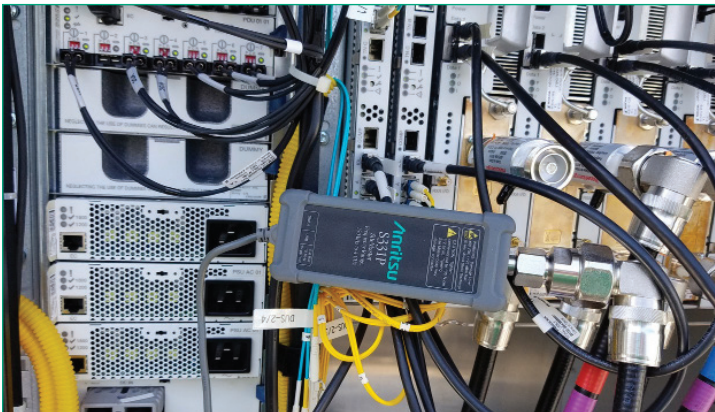
Direct connection to DUTs
